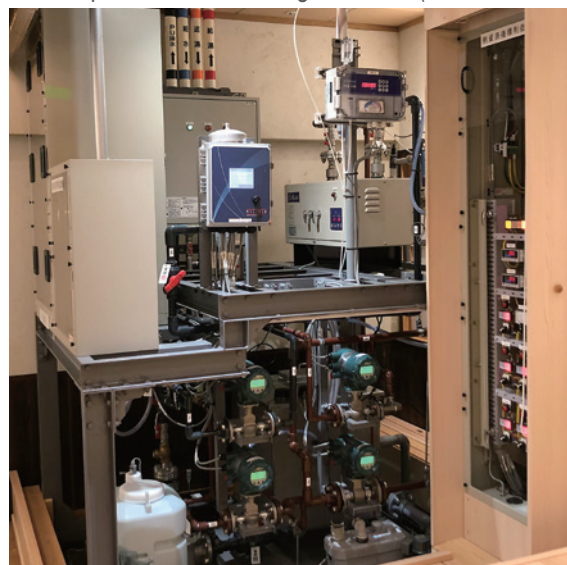
Thermal Resource Circulation Plant
