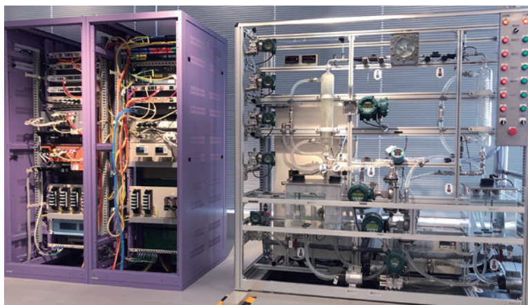
Thermal Energy Conversion Plant
