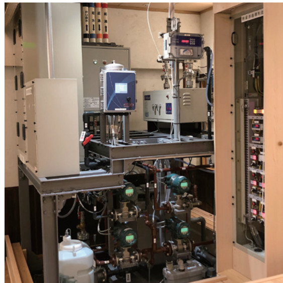
Thermal Resource Circulation Plant
